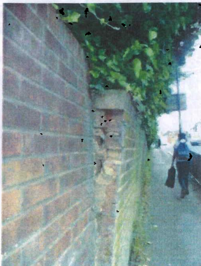
Photo No. 02 – Lean outwards as at June 2014
