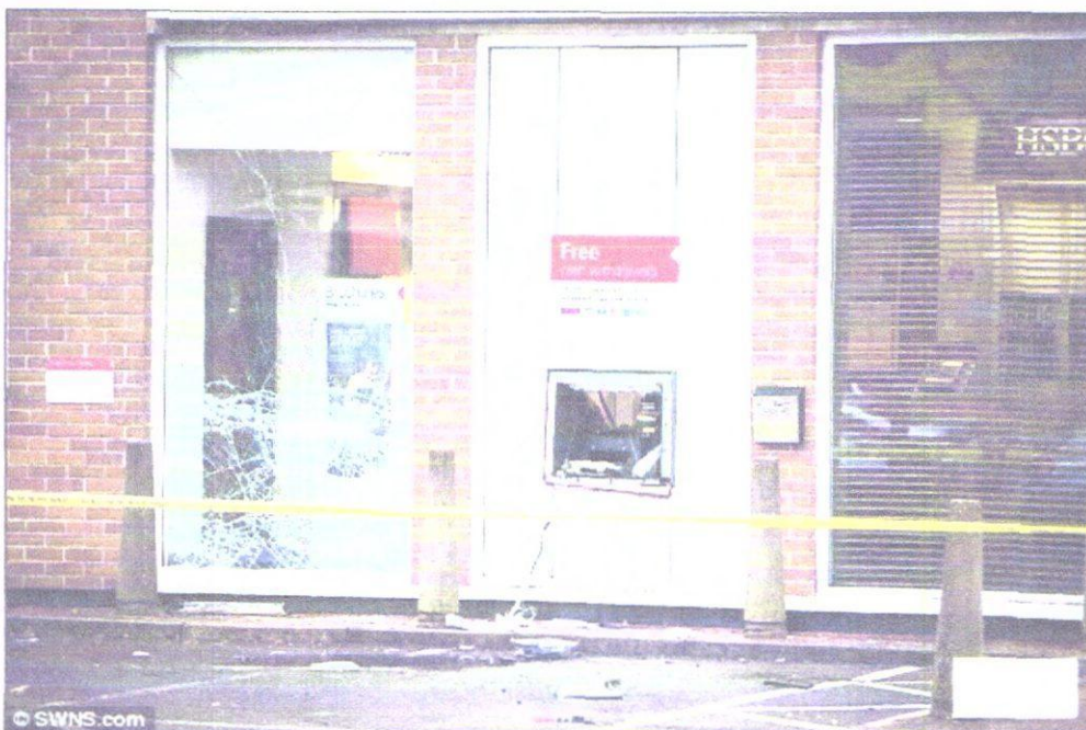
A glass window was smashed in the blast and thieves in dark clothing escaped with thousands of pounds
