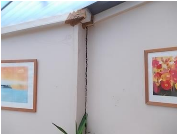
FIGURE 03 Verical crack on RHS of conservatory.
