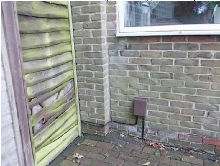
FIGURE 05 cracks on front elevation below kitchen window
