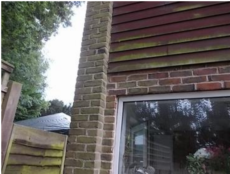
FIGURE 06 Diagonal crack above kitchen window
