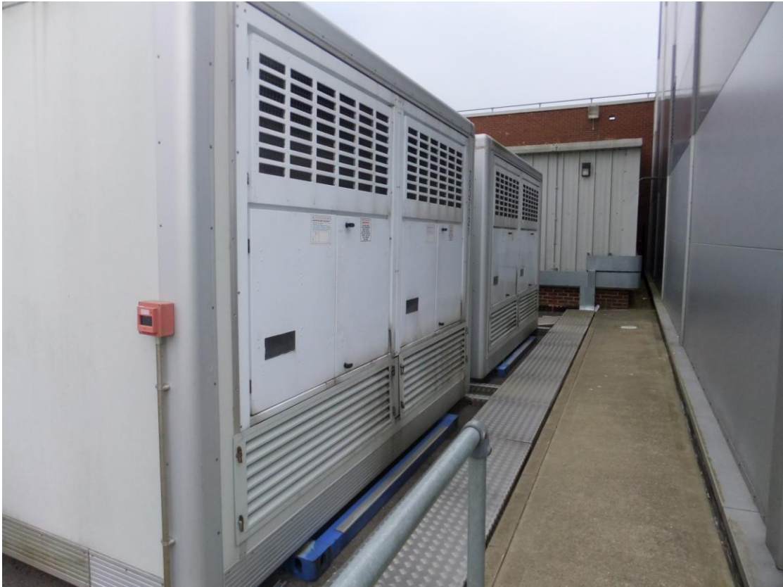
Photo 1 View of the chillers of the older existing freezers
