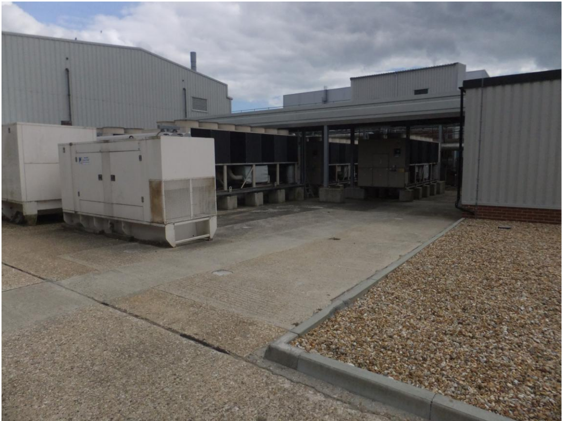
Photo 2 A bank of chillers located close to HPS car park on north boundary
