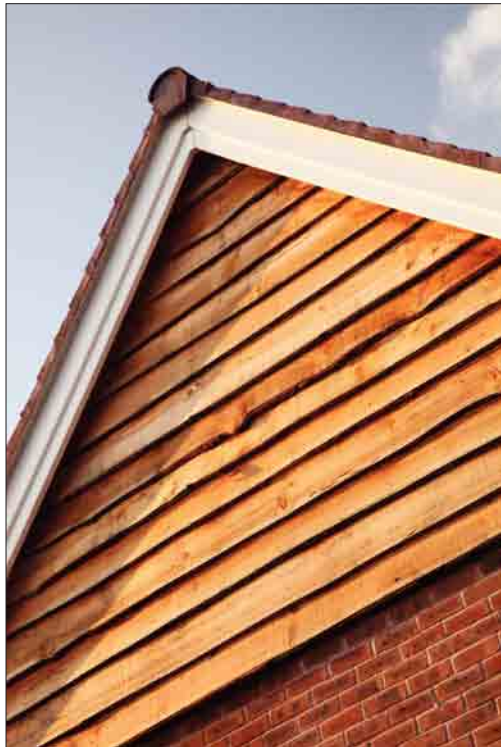
Photo 4 : Wavy edge boarding on garages
