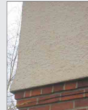
Photo 8 : Render to brick bellmouth detail on Arts and Crafts cottages at Greenhill Road, Winchester
