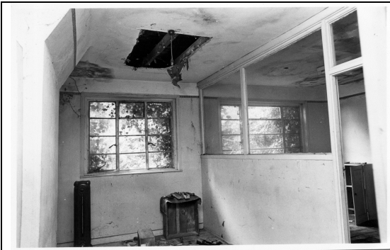
5-Photograph showing the state of the structure when our client purchased the building in 1979
