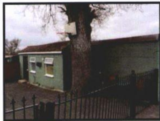
Image 3: Tree 4 growing directly adjacent to one of the existing outbuildings with hard surfacing located up to the base.
