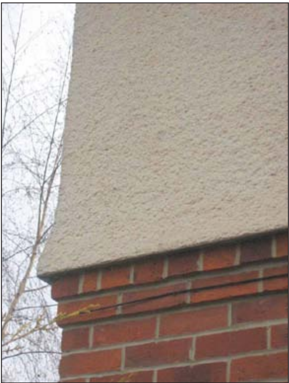
Photo 1 : Render to brick bellmouth detail on Arts and Crafts cottages at Greenhill Road, Winchester
