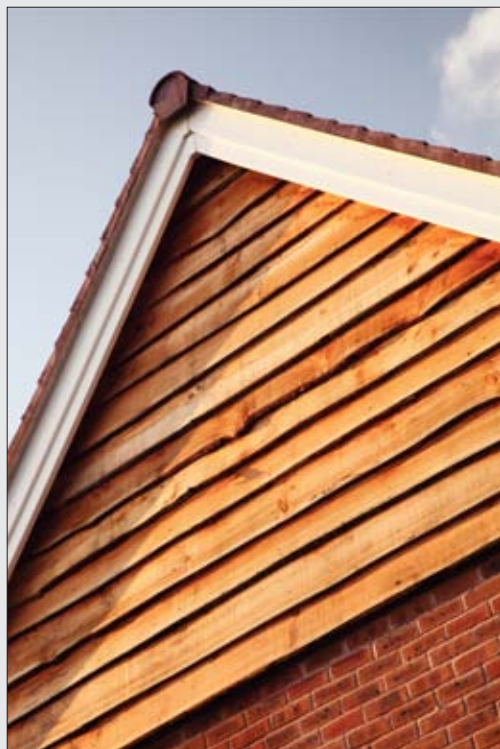
Photo 6 : Wany edge boarding on garages
