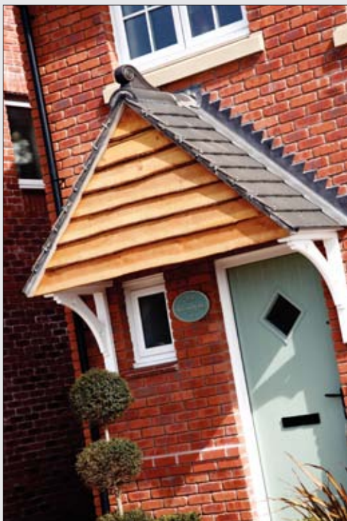
Photo 7 : Wany edge boarding on porches
