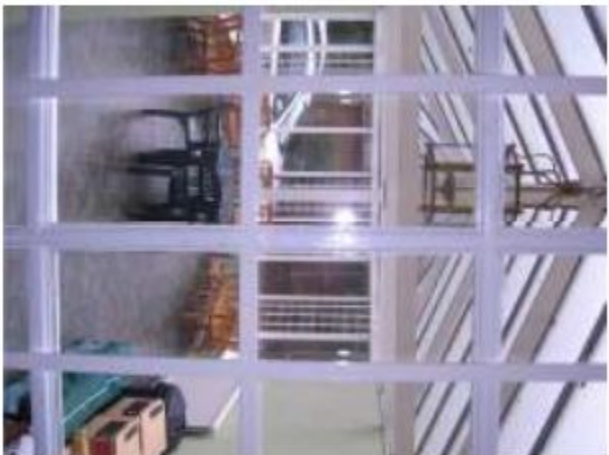
d - looking inside the conservatory: poorly insulated, this recent addition is proposed to be replaced with a new timber framed conservatory
