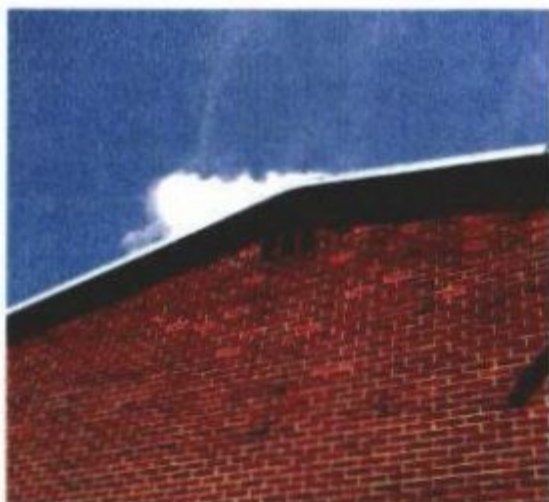
Figure 2. Apex air grille in the west-facing gable end of the south Junior School building
