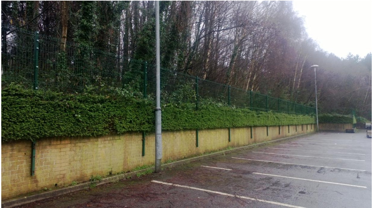
Photo 1. Showing area of retaining wall affected by development
