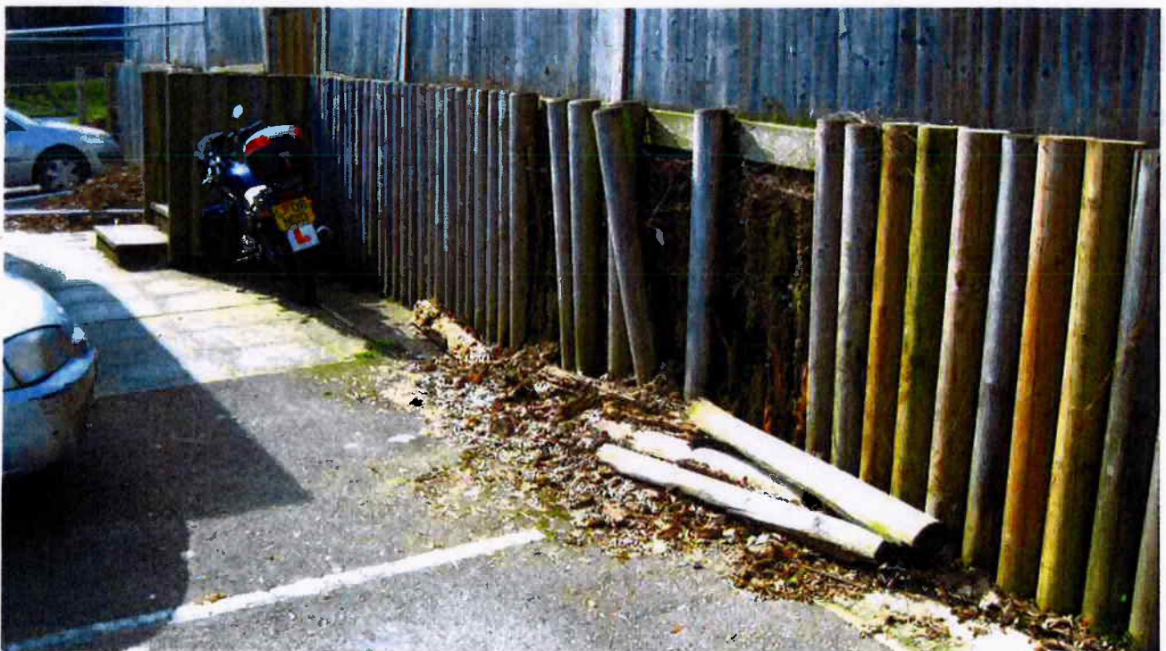
Photograph B – View of the failing timber posts.
