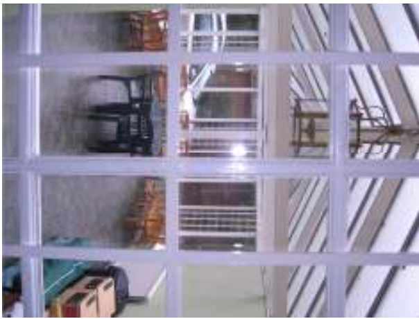
d - looking inside the conservatory; poorly insulated, this recent addition is proposed to be replaced with a new timber framed conservatory
