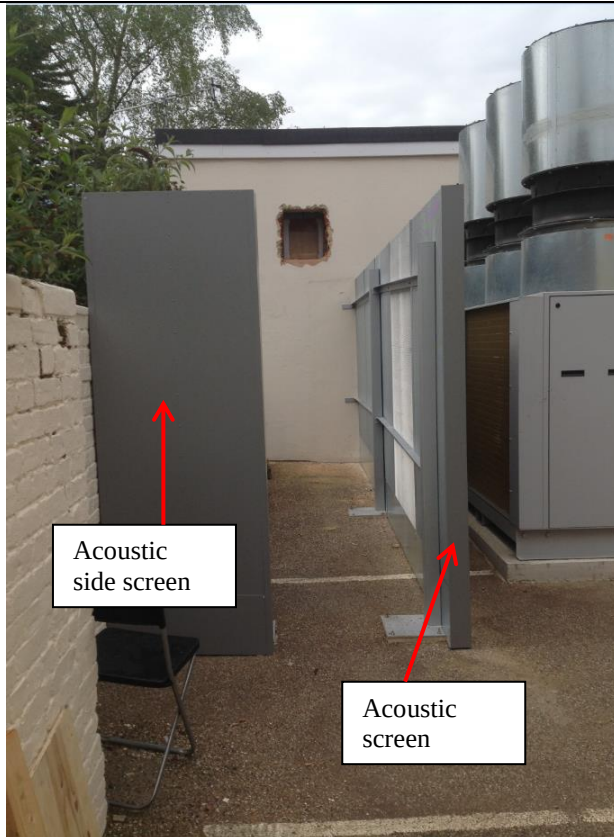
Figure A1. Condenser an acoustic screen (prior to the installation of hit-and-miss fence and ACs)
