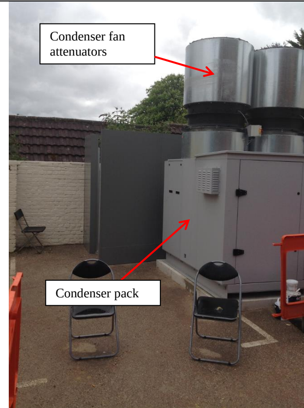
Figure A2. Condenser an acoustic screen (prior to the installation of hit-and-miss fence and ACs)
