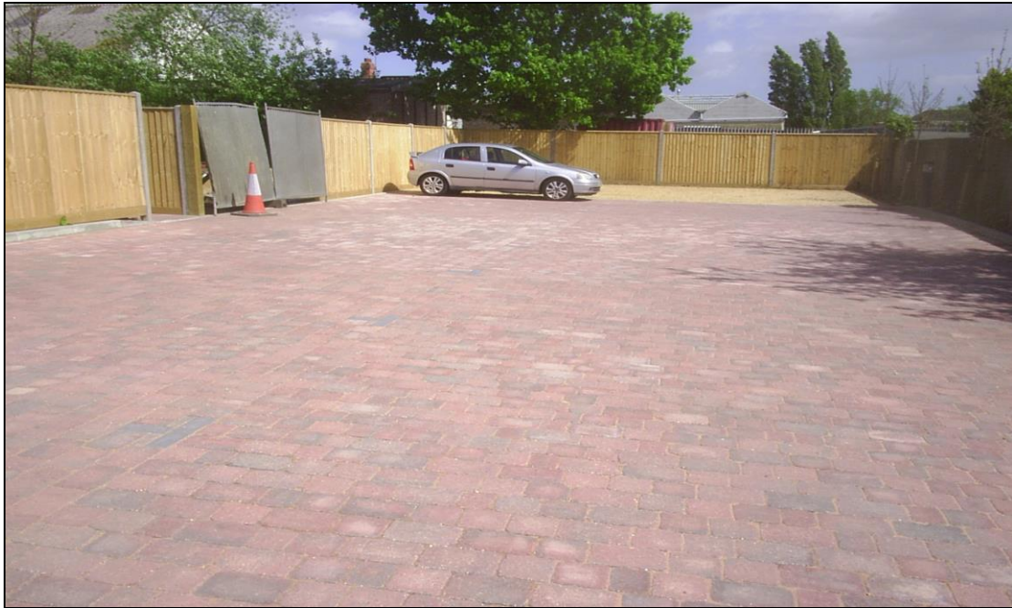
Photograph 8 Showing the ground slope in the car park
