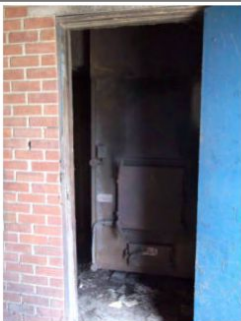
Photograph Five – Boiler room, Unit 25d
