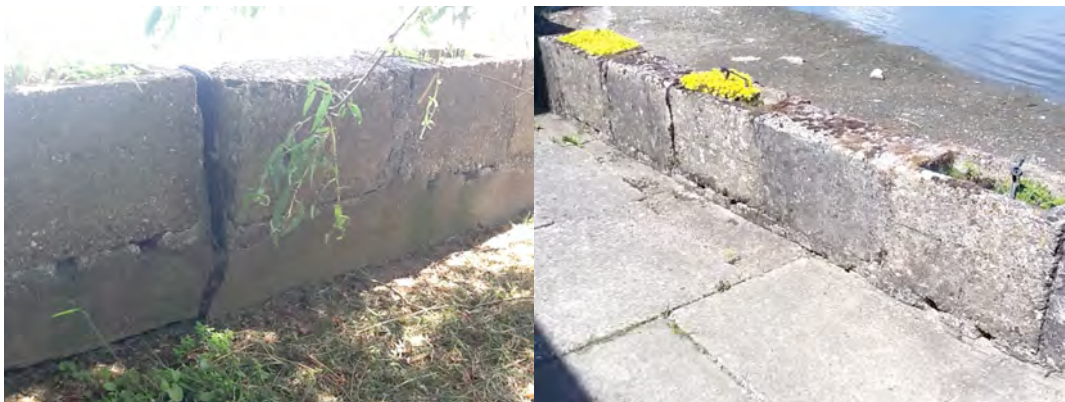
Fig 2 Eroded sea walls
