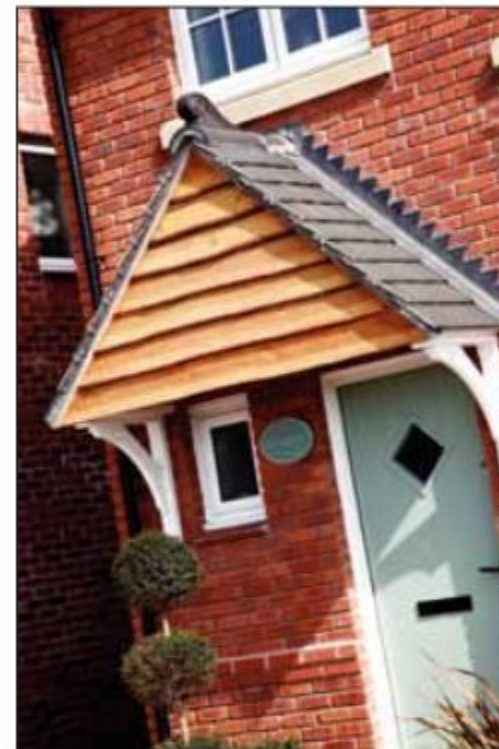
Photo 5: Wany edge boarding on porches
