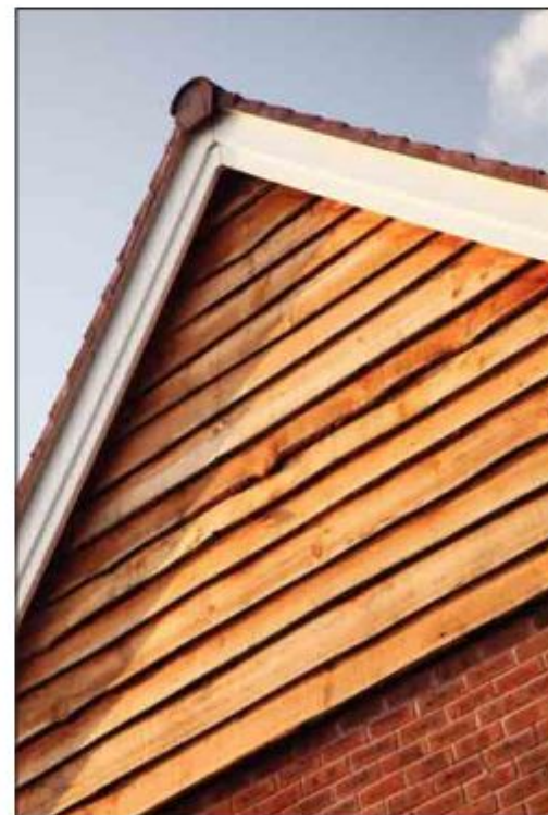
Photo 4: Wavy edge boarding on garages
