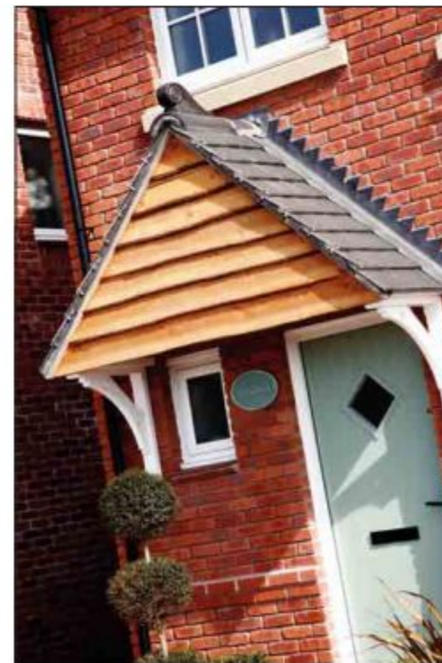
Photo 5: Wavy edge boarding on porches
