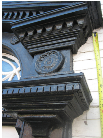
Fig 3 - Existing detail of the dentilled pediment and broken cornice above pilasters
