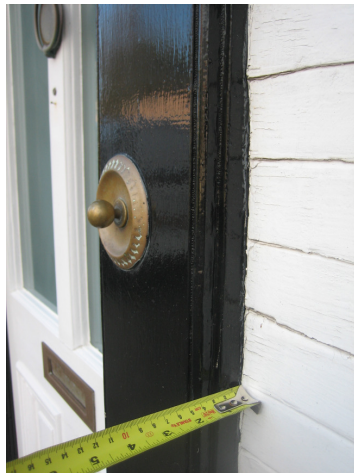
Fig 2 – Existing door surround projection from the cladding facade
