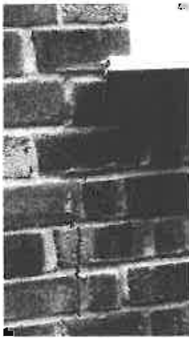
Crack on left hand flank, below window
