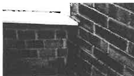
Crack below bay
