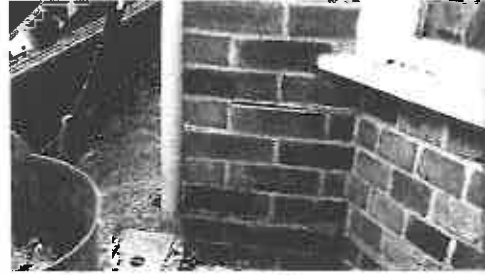
Crack at rear right hand corner
