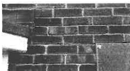
Crack to side of bay at high level
