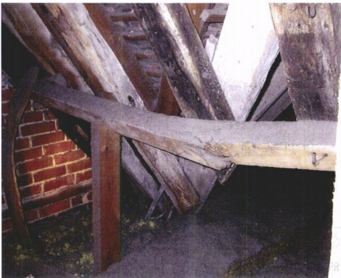
Photo 017 – S.W. Roof Space. Rear Pitch. Broken Lower Purlin.
