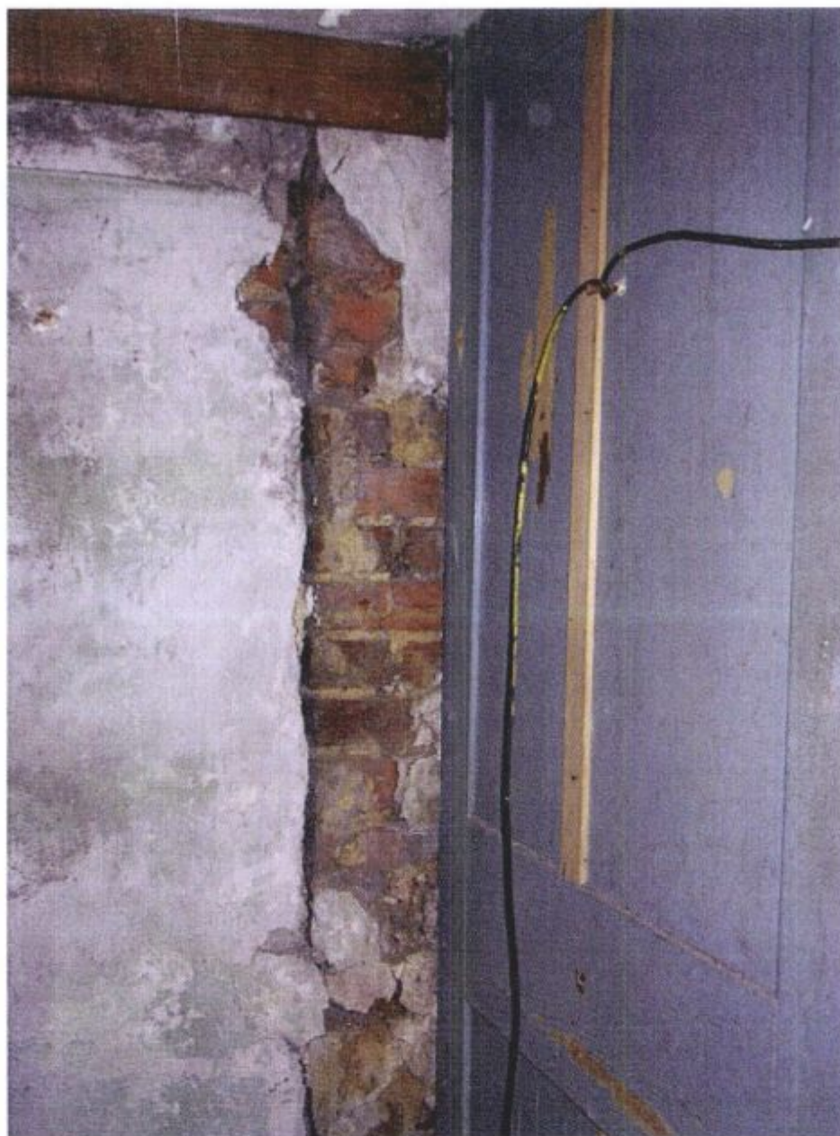
Photo 027 – Bedroom 2. S.E. Corner. Party/Front Wall Junction.
