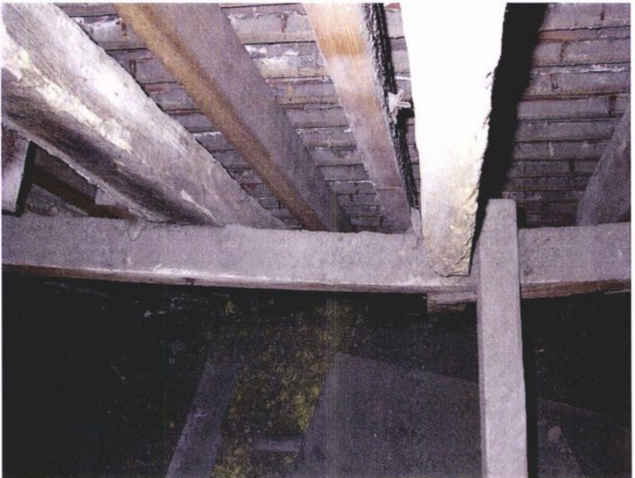
Photo 012 – S.W. Roof Space. Front Pitch. Broken Purlin at Strut Position.
