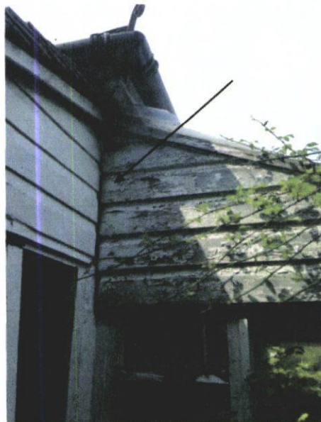
Fig 3) Kitchen area meeting conservatory/potting shed showing cobweb covered gaps.
