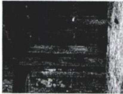
Figure 6 Gaps within Ridge Tiles
