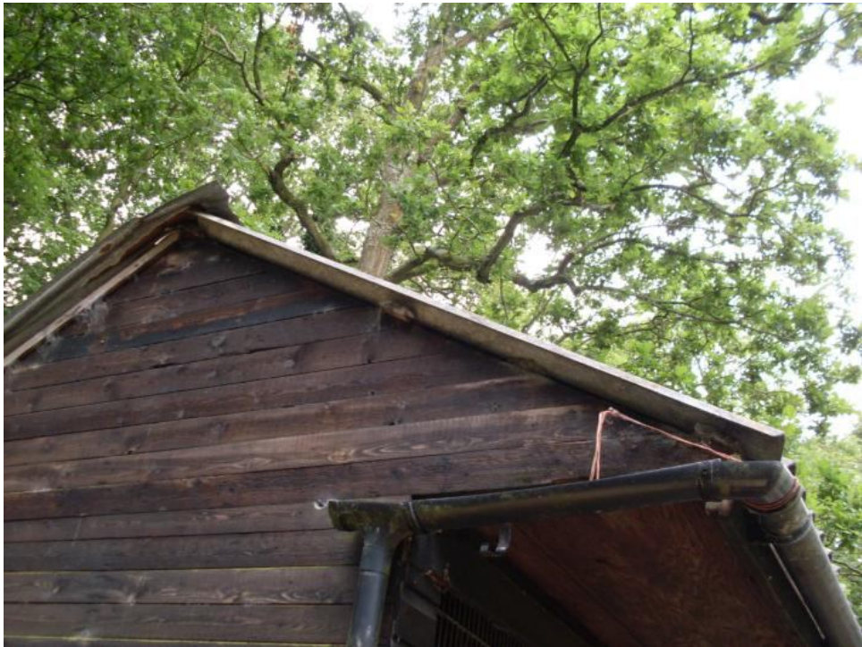
Gap between timber cladding
