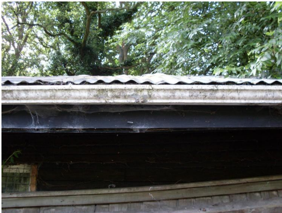
Gap between the corrugated roof and the timber boards below
