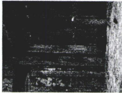
Figure 6 Gaps within Ridge Tiles
