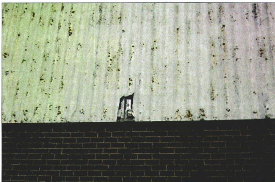
Photo 1 – hole to external cladding showing metal internal cladding
