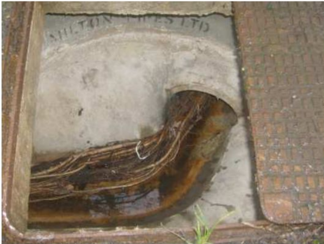
ROOT PENETRATION INTO EXISTING STORM SEWER AT MANHOLE A
