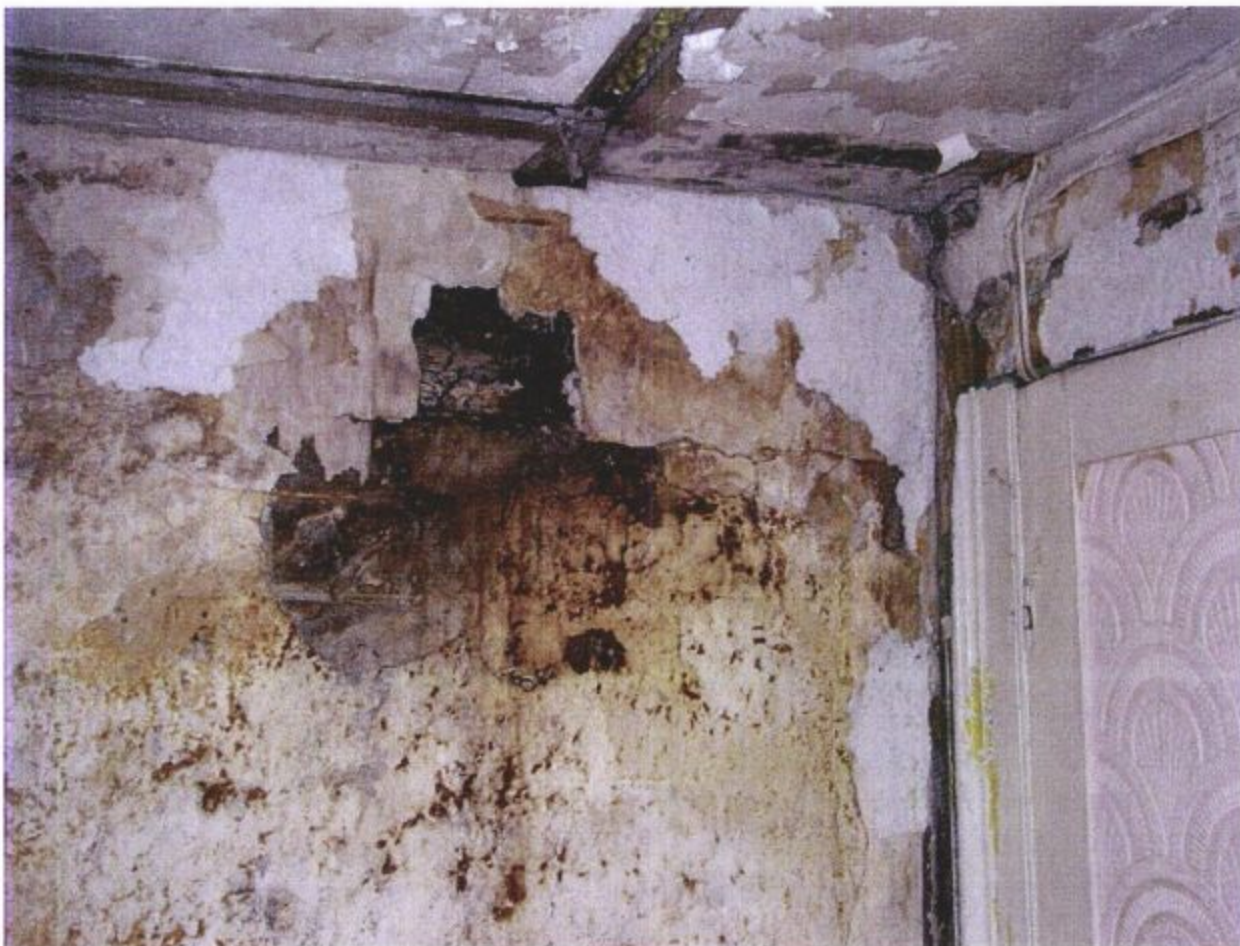
Photo 026 – Bathroom S.W. Corner. Bedroom 3 Partition. Timber Frame Decay.
