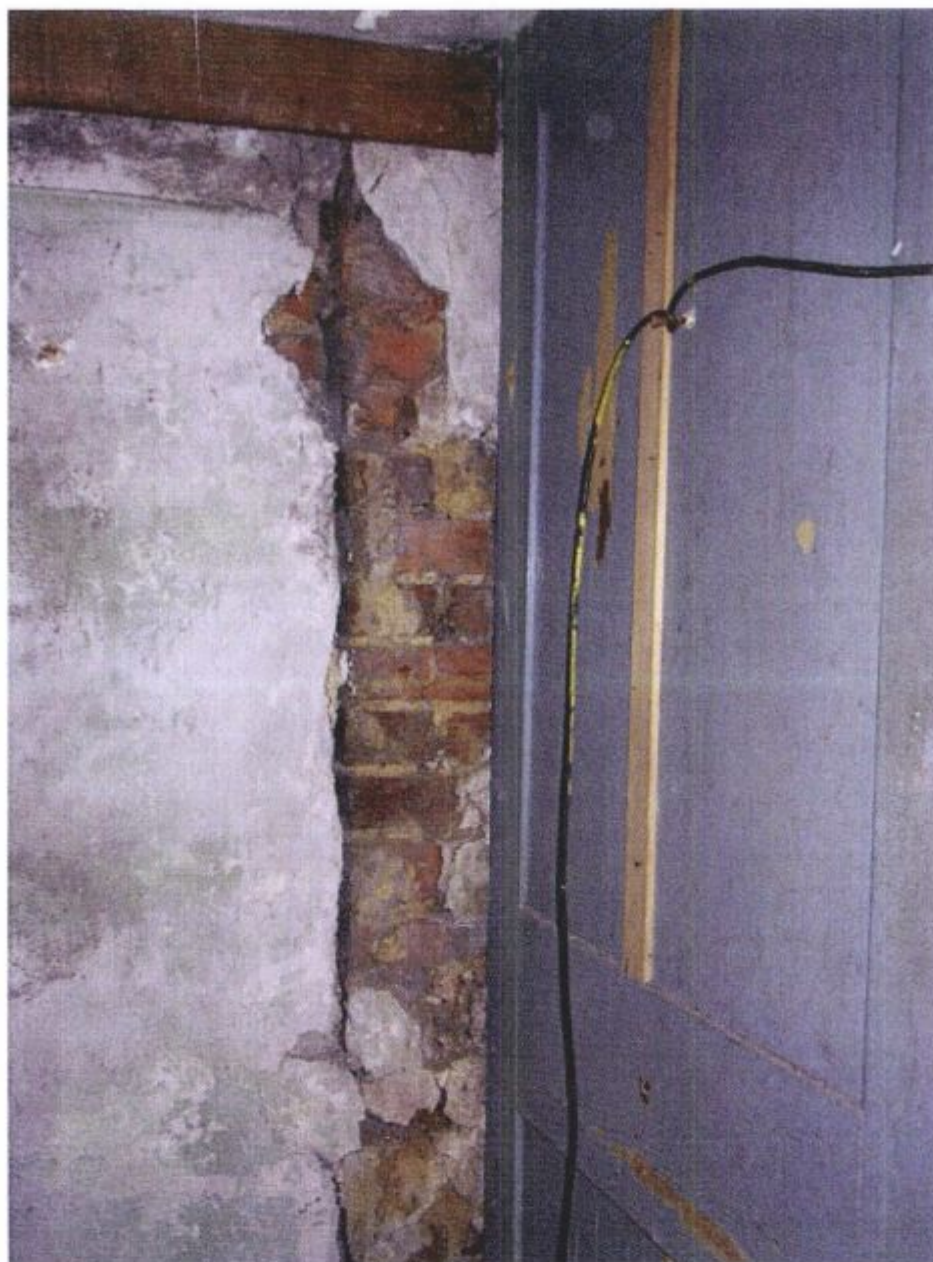
Photo 027 – Bedroom 2. S.E. Corner. Party/Front Wall Junction.
