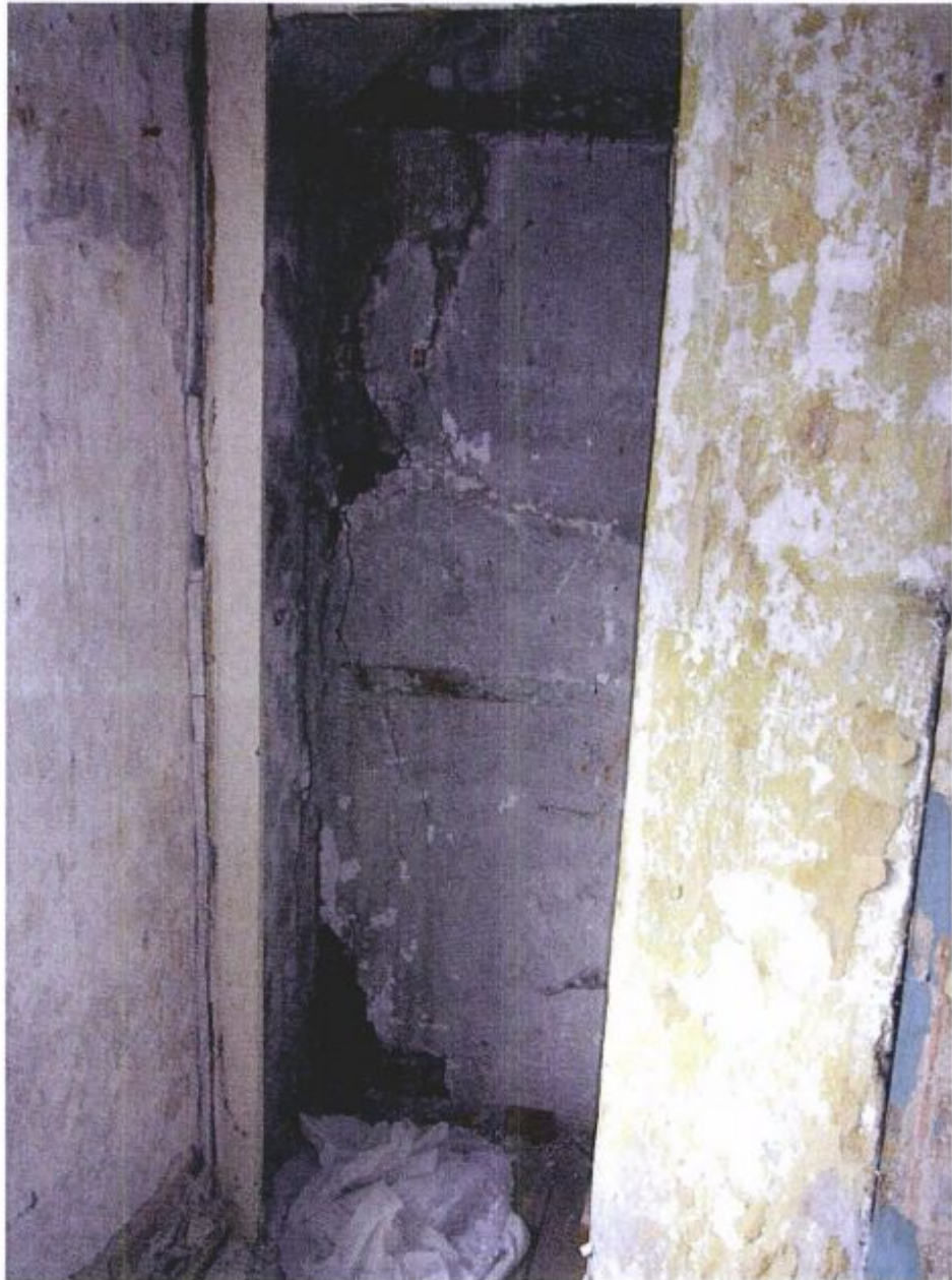
Photo 023 – Bedroom 1. S.W. Corner. Junction of Front Wall and West Party Wall.
