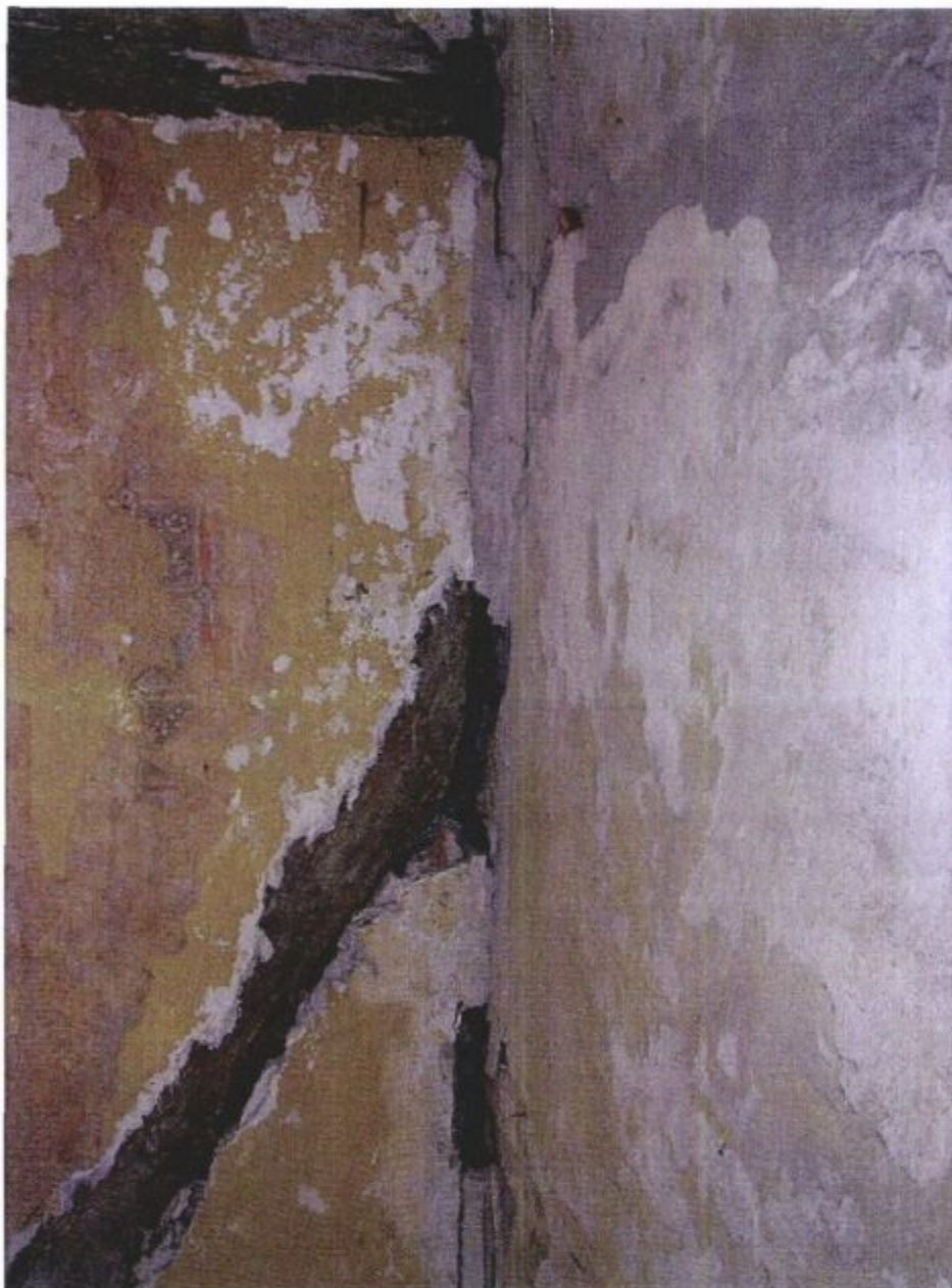
Photo 019 – Bedroom 1. S.E. Corner. Partition/South Wall Junction.
