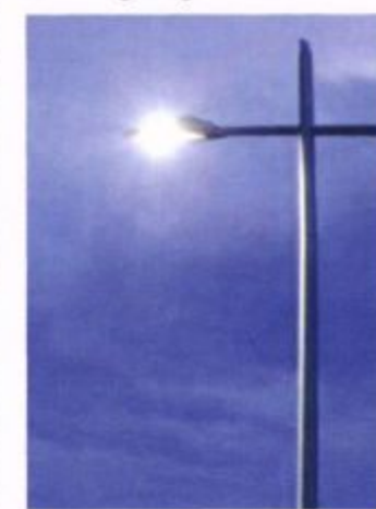
Street lighting - columns
