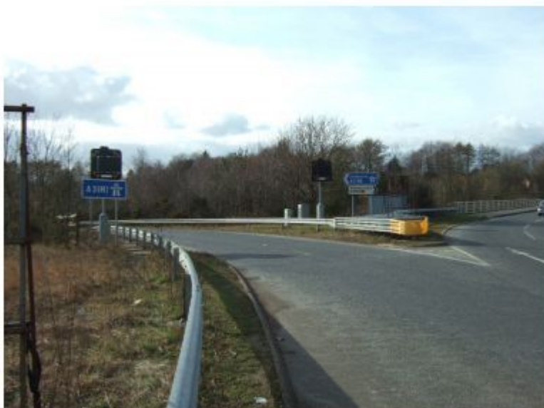
Figure 2. Crash Cushion at A3(M) Junction 3 Southbound On-slip
