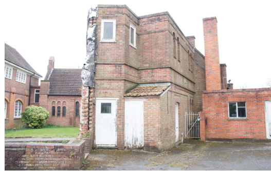
Badly patched remains of the two storey building and boiler house at the north east nave of the church
