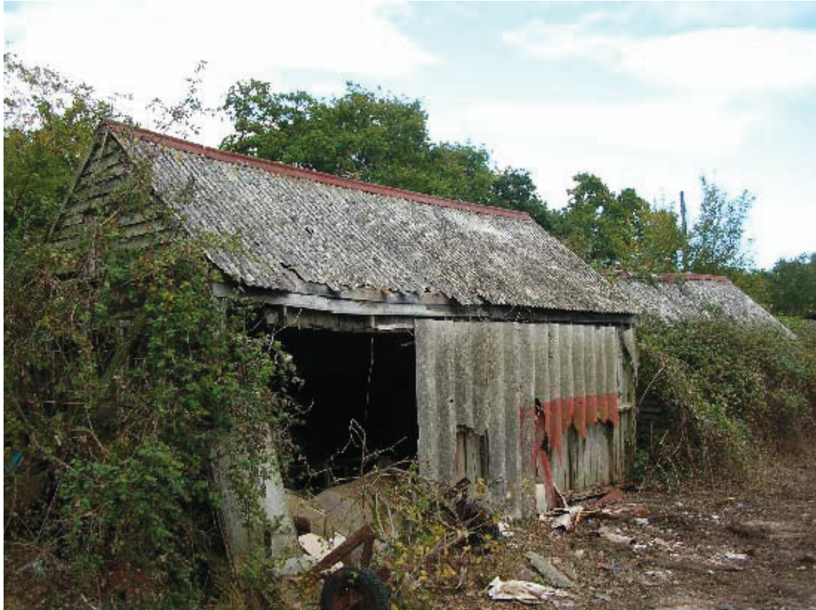
Photo 3 - Shed with gap between asbestos roof and internal cladding, potential for bats
