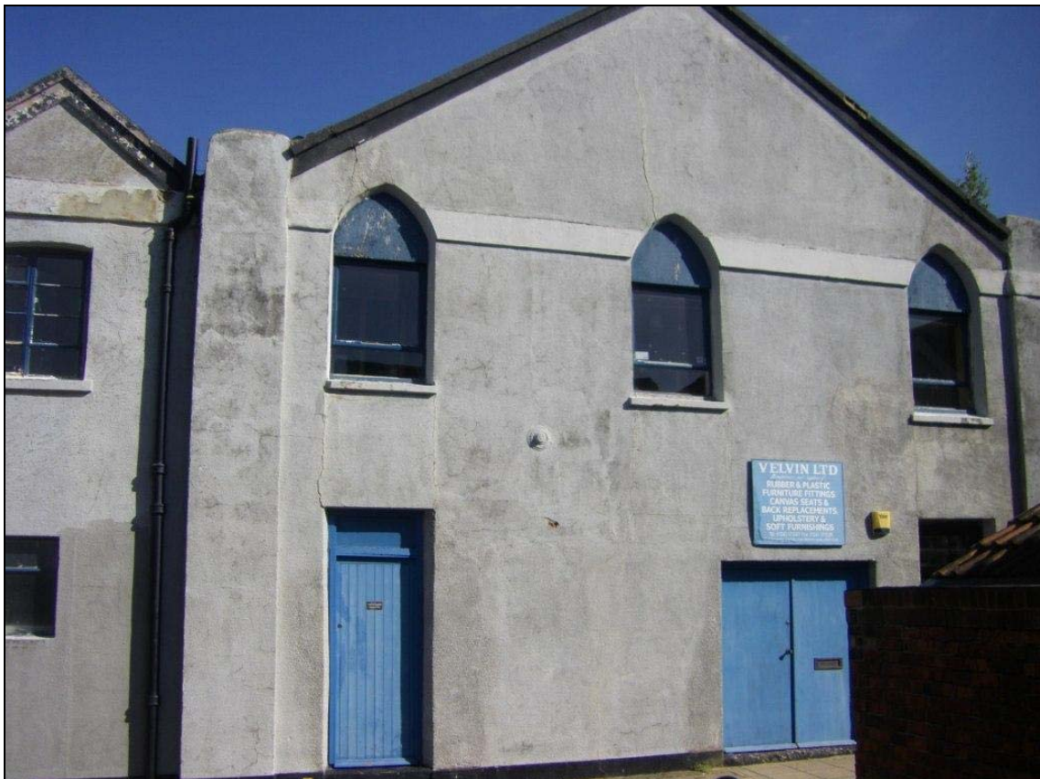
Photo 1: Front elevation, cracking on wall visible
