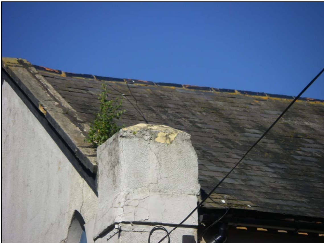
Photo 2: East pitch of the roof with capped gable upstand wall and vegetative growth. The slates are in a poor condition. There is no underfelt or insulation.
