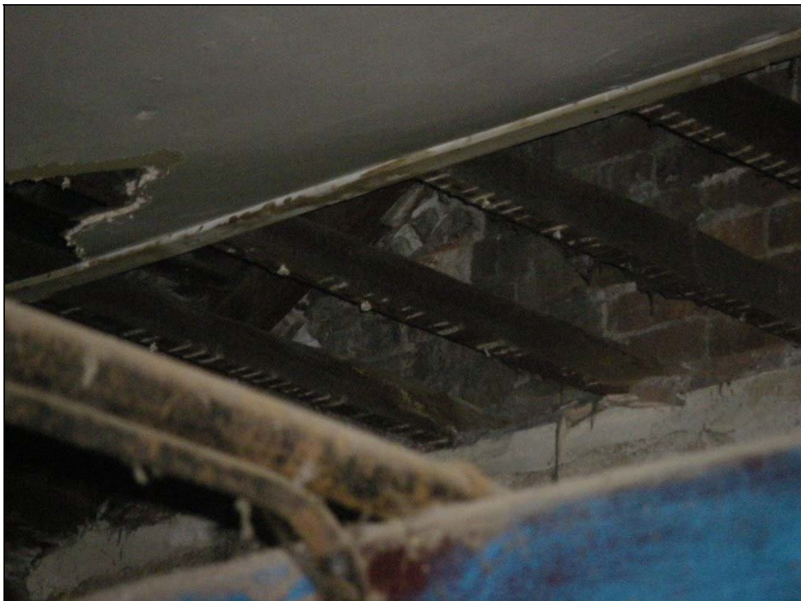
Photo 7: Lath and plaster missing from ceiling joist on first floor. The ceiling joist where supported by a wall can provide lateral restraint however if the timber decays the effectiveness of the lateral restraint will be compromised.
