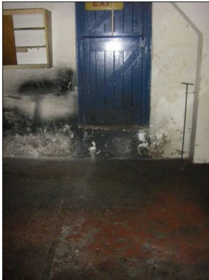
Photo 5: The external ground level is at the bottom of the door. There is dampness both on the walls and floor.
