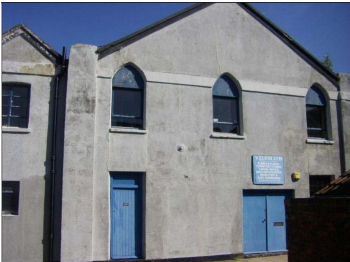
Photo 1: Front elevation, cracking on wall visible
