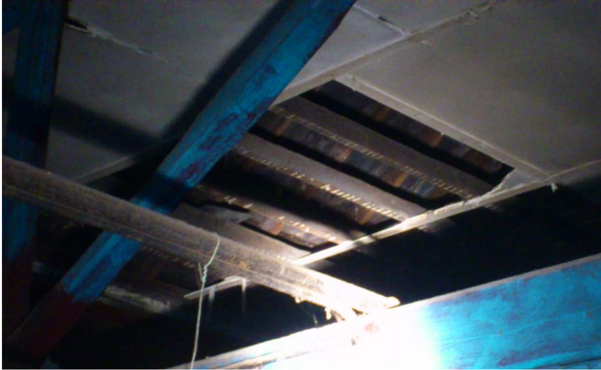
Photograph No. 15 - Missing panels exposing roof void. It can be seen that there is no roof membrane that will reduce the potential for viable bat roost space within the loft void, and equates to 'Negligible' Bat Roost Potential.
