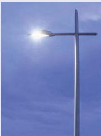
Street lighting - columns
