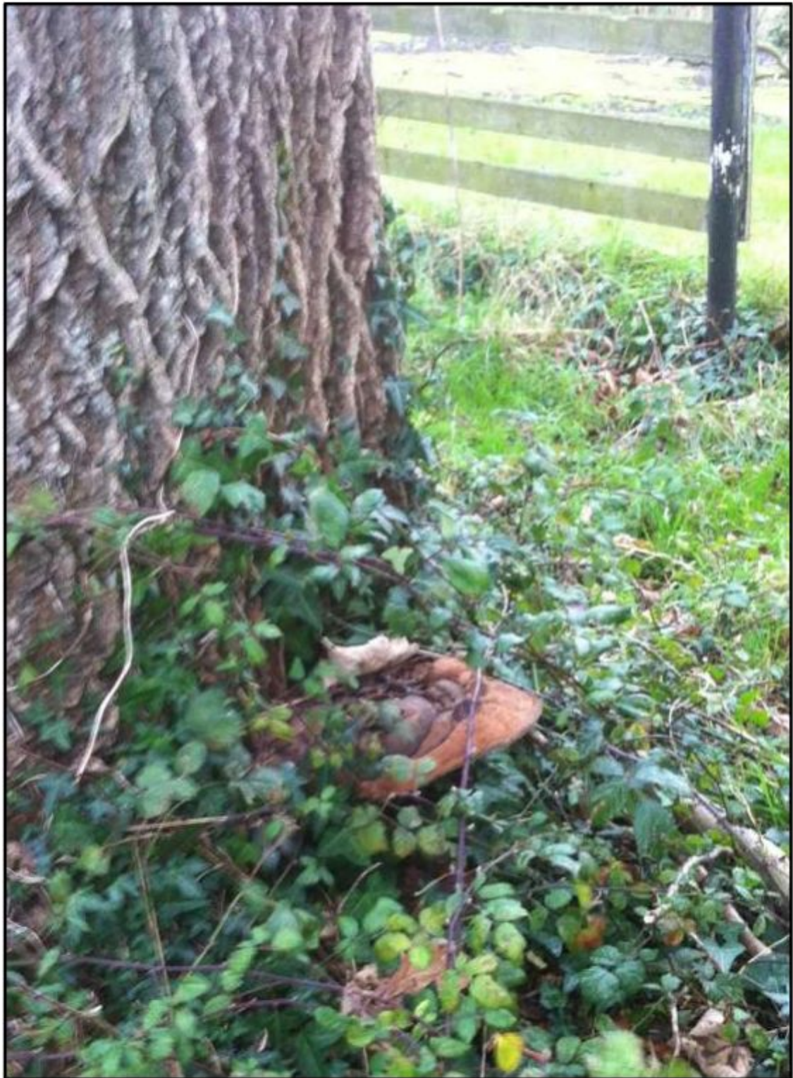
Photo 2: Close up detail of bracket fungus ( Ganoderma sp) observed at the base of tree 41 (southern side).
