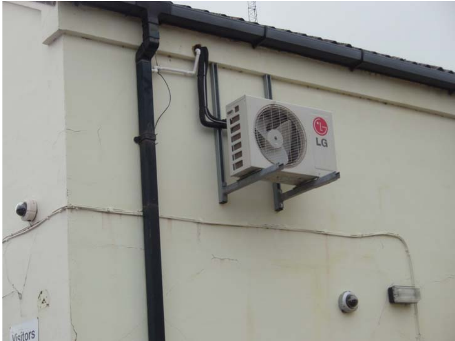
Photograph 2 – Air condenser on the reception building.
