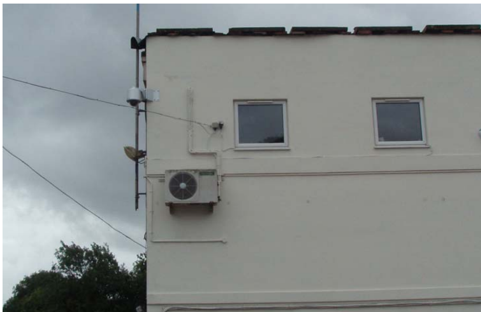
Photograph 3 – Air condenser unit on the north elevation of the office/workshop building.
