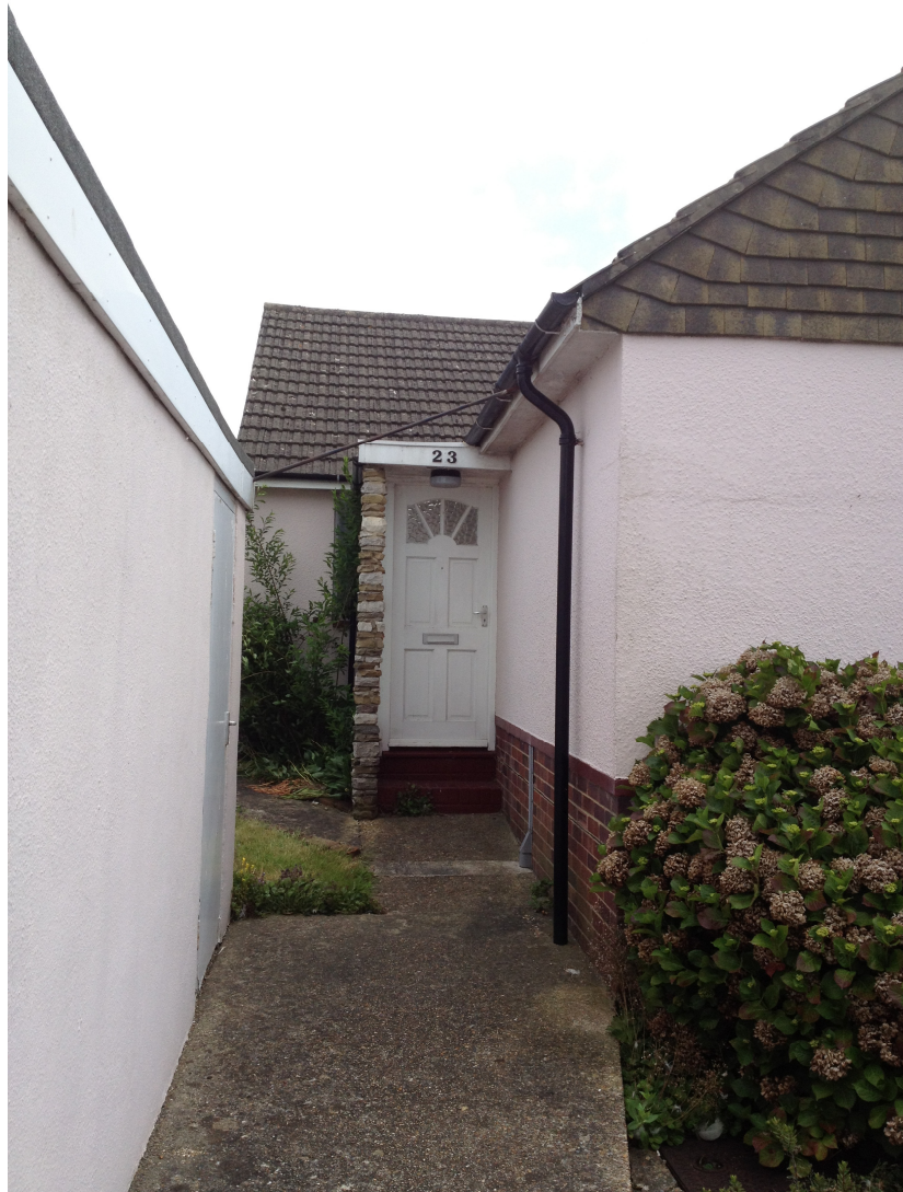
Fig 3: Existing Dilapidated Porch
