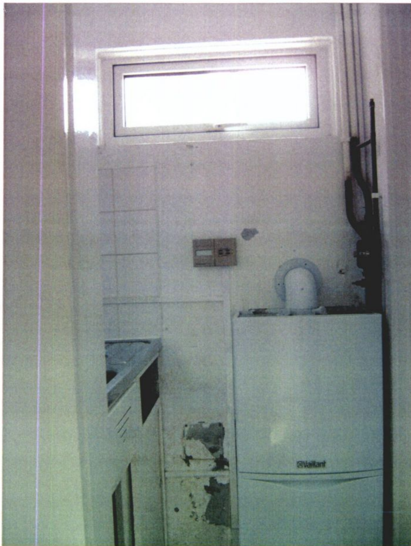
Interior of existing building showing central heating boiler and cloakroom
