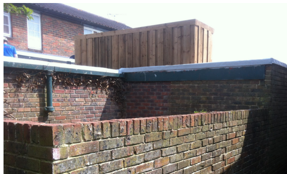
Figure 3: Photograph of Extract Flue
