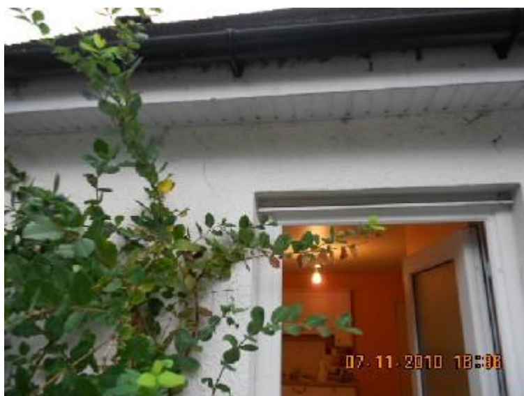
FIGURE 6 Thermal cracking around the end of the lintel bearing above the left hand kitchen door
