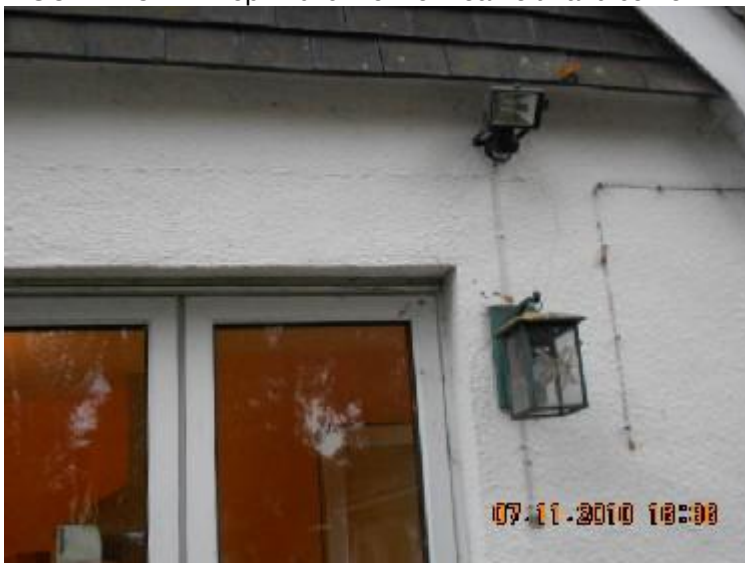
FIGURE 5 Thermal cracks around lintel bearing at the rear kitchen window
