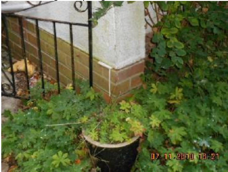
FIGURE 4 8mm Drop in brickwork on rear left hand corner
