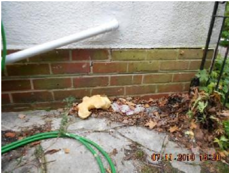
FIGURE 3 Diagonal tapering fracture in the brickwork at low level
