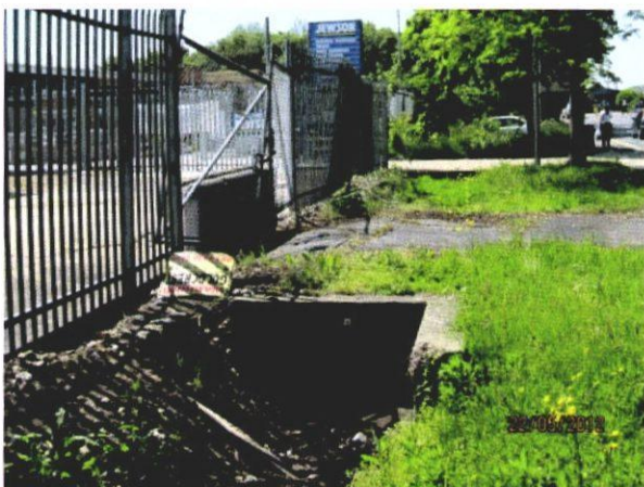
Partially blocked crossing
