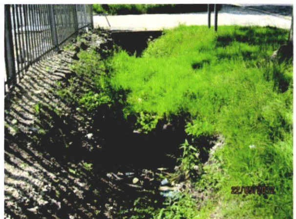
Partially blocked crossing
