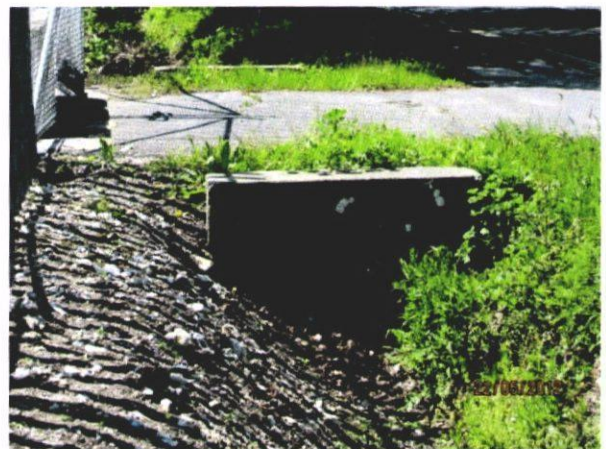
Partially blocked crossing
