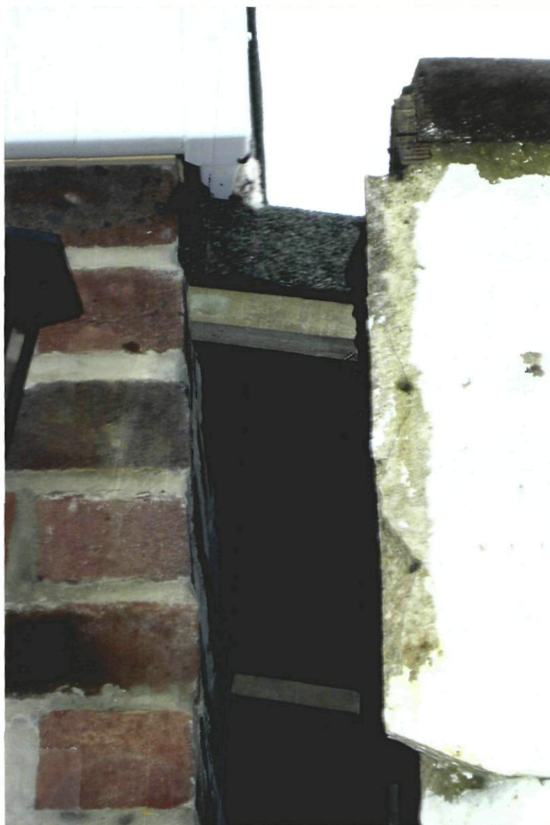
PHOTO 5 - DIRECTION (A) ON 1:500 OS MAP THIS VIEW SHOWS THE FLAT ROOF BRIDGING MINE AND MY NEIGHBOURS GARAGE
