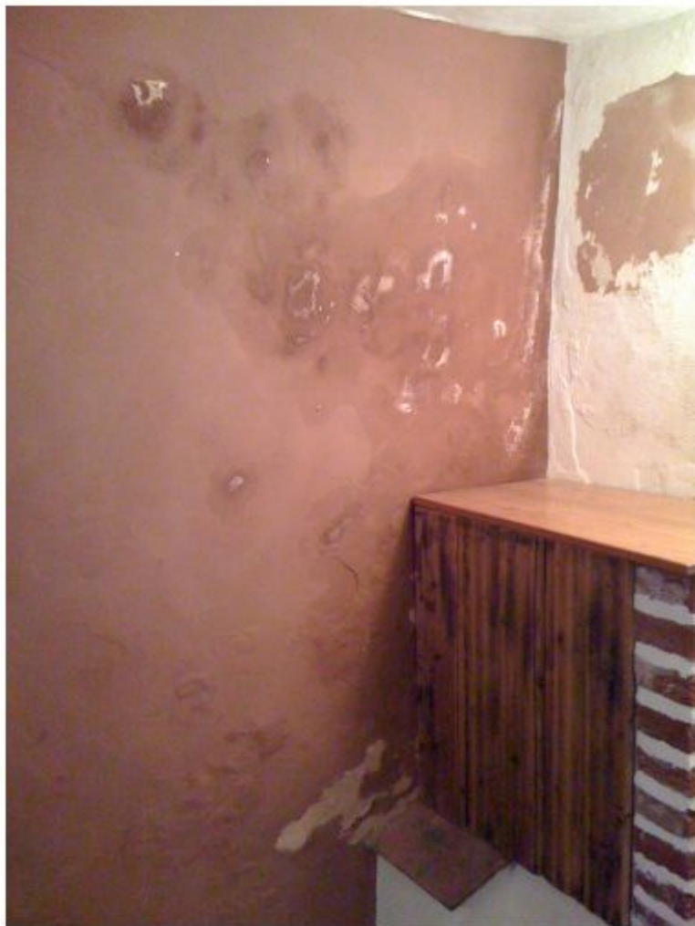
8 Langstone High Street: photographs of damp we are trying to prevent or isolate from interior.
