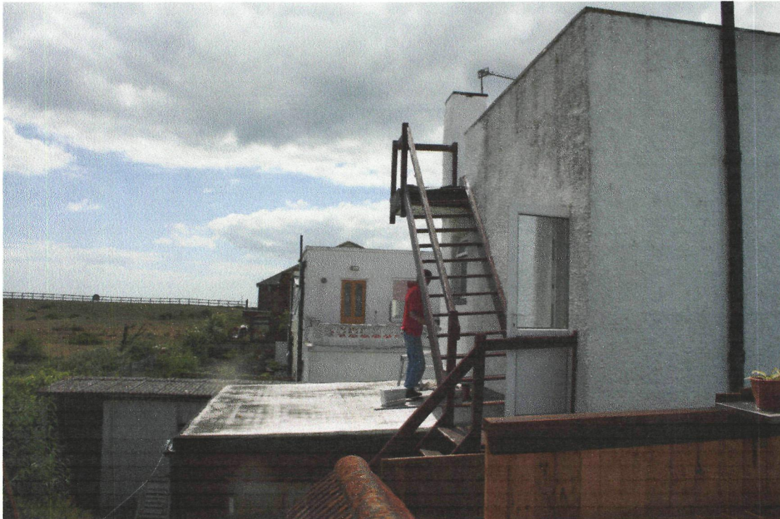
25 Sandy Beach Area showing the unsafe stairs access to ground and roof, outside decking area and use of roof area all these overlook 24 Sandy Beach Estate. Beyond this is 29 Sandy Beach Estate (next door to 25 Sandy Beach Estate) showing outside area used on the side of the building.
