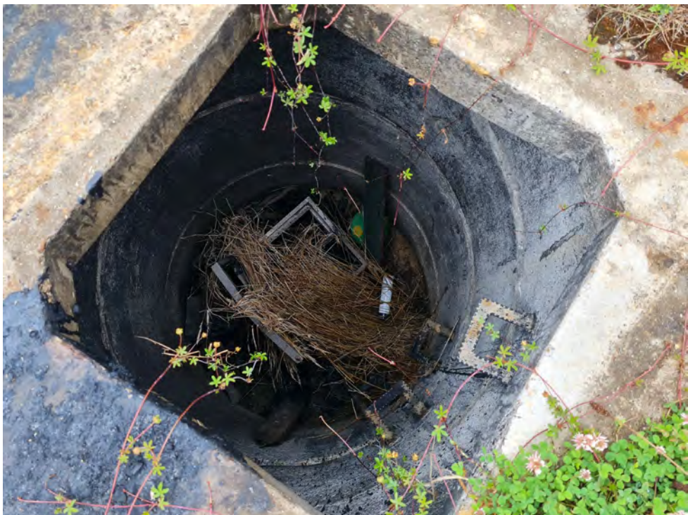
Plate 8: Rubbish was observed inside one (above), brick and concrete rubble in the other.
