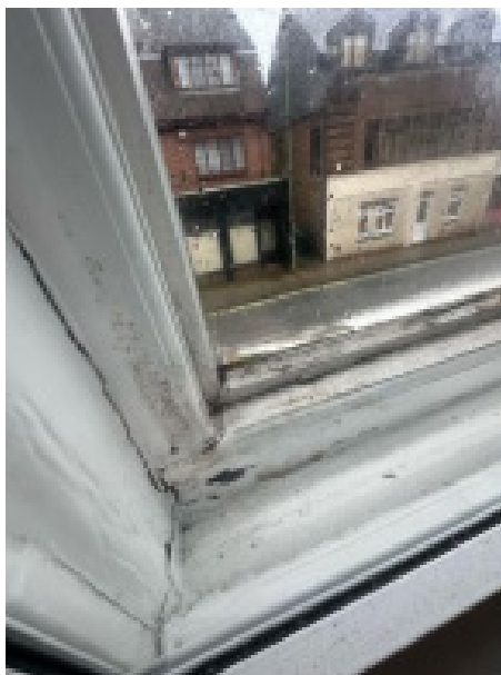
Image 03 Rotting condition of existing timber window frames.
