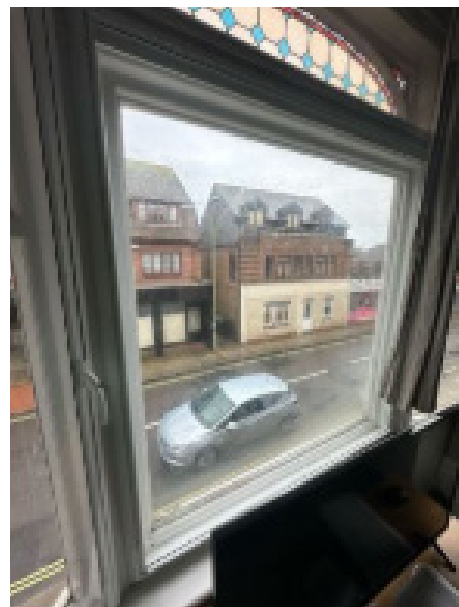
Image 04 Poor condition of bay window frames.
