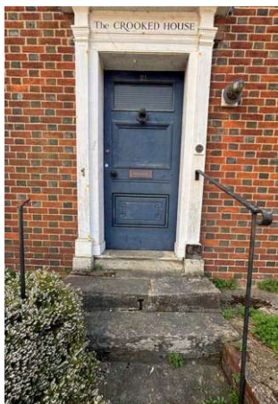
Figure 69: Front doorstep & surround to be repaired.
