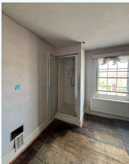
Figure 54: Shower to be removed.
