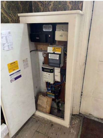
Figure 35: Existing Location of Electric Meter
