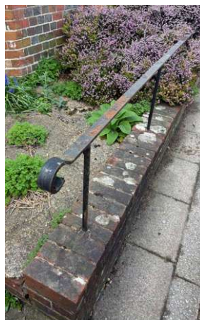
Figure 71: Railings to be repaired.
